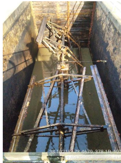
Broken flocculator shaft
